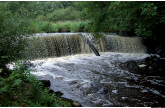
Severnaces Weir, Ayrshire, Scotland Main constraint: Potential for extensive upstream channel adjustment Option recommended: Partial removal with informal fish easement
