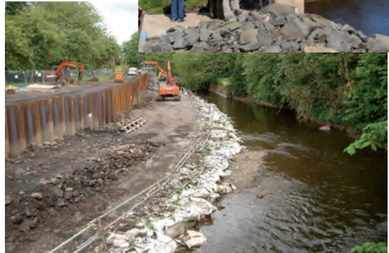
Inlet to flow control structure at Kirkland Bridge storage area (above) and flood wall under construction in Cathcart .
